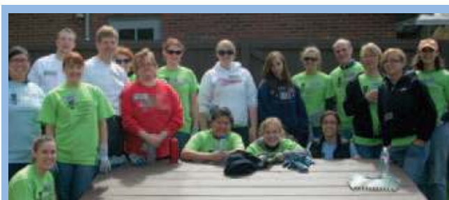
Over 60 Rebuilding Together Seattle volunteers gave the campus a makeover in April by renovating gardens, building a fence, installing new lighting and much more.
